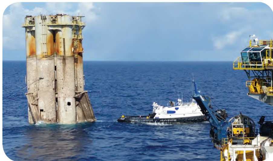
Top: With holes cut into the hull, Red Hawk spar is being tipped underwater. Above: Red Hawk Spar was towed vertically to its reefing site. Images from InterMoor.
