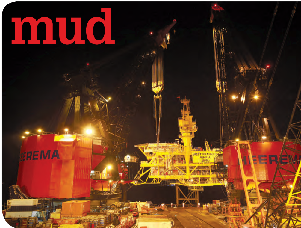
The West Franklin well head platform installation last year. Photos from Total.
