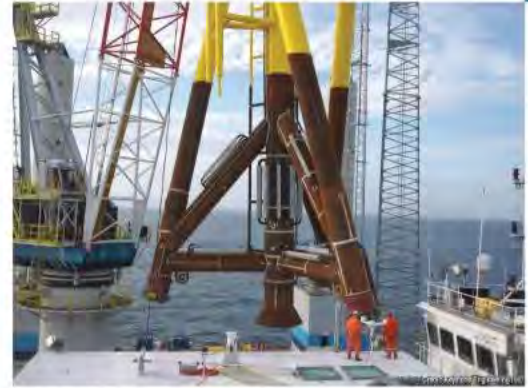
The twisted jacket foundation upright. Photos from Keystone Engineering.
