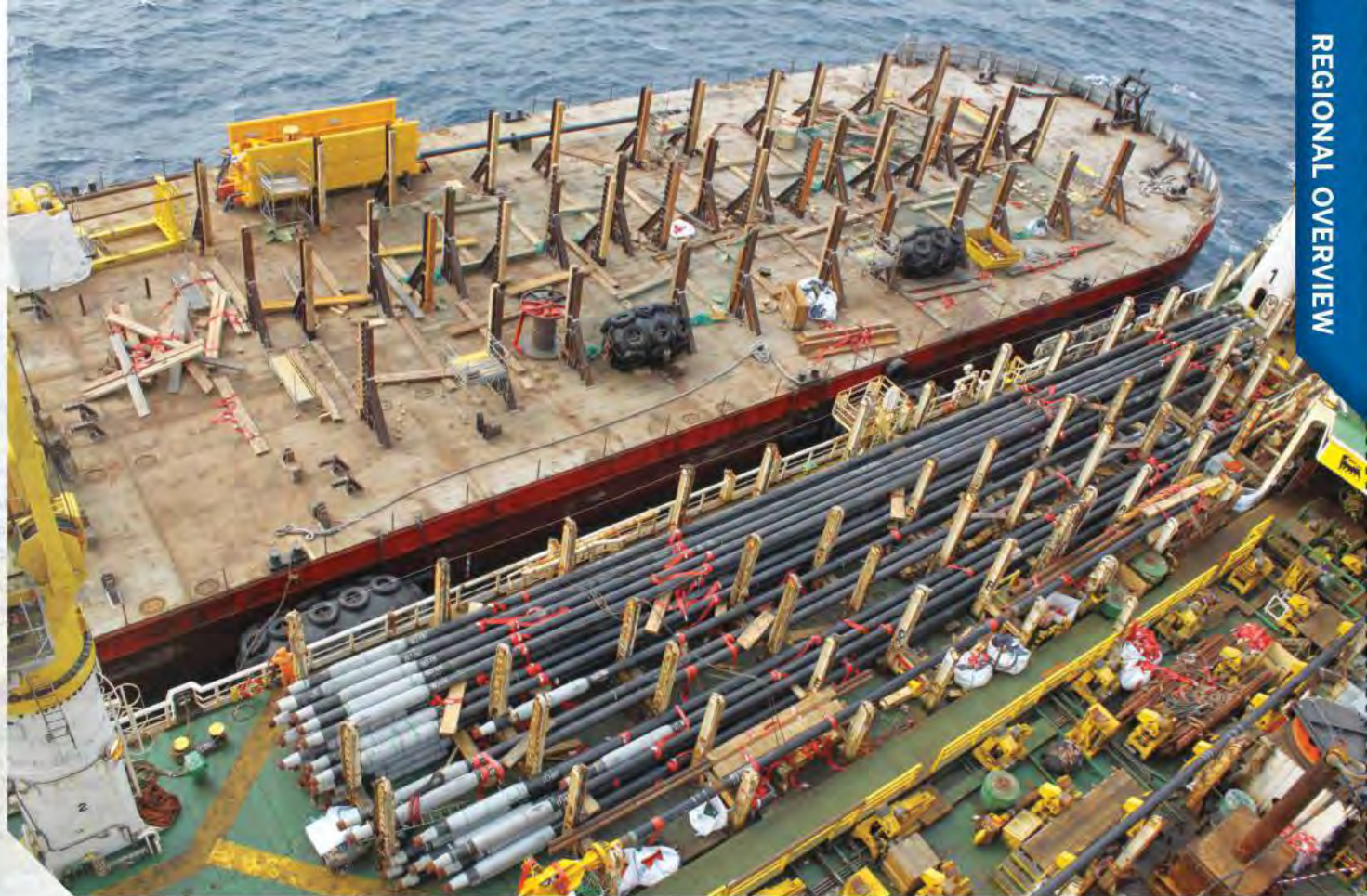
Hundreds of pipelines are transferred by crane from a cargo barge to the vessel that lays them on the sea bed at Bonga North West offshore oil field.
