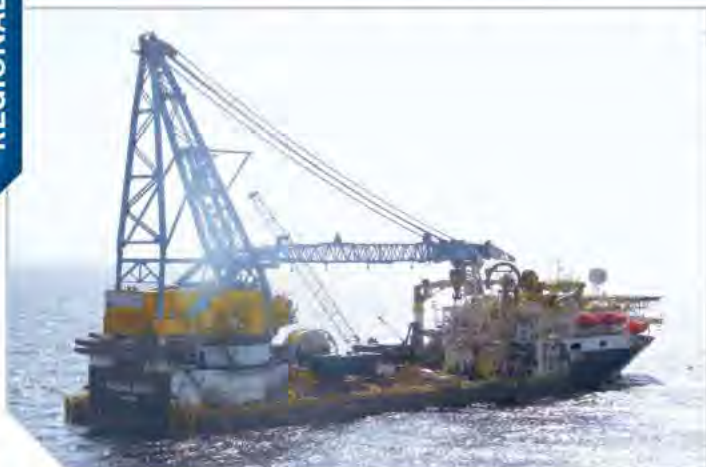
The Saipem 3000 vessel installs umbilical cables at the Bonga North West offshore oil field.
