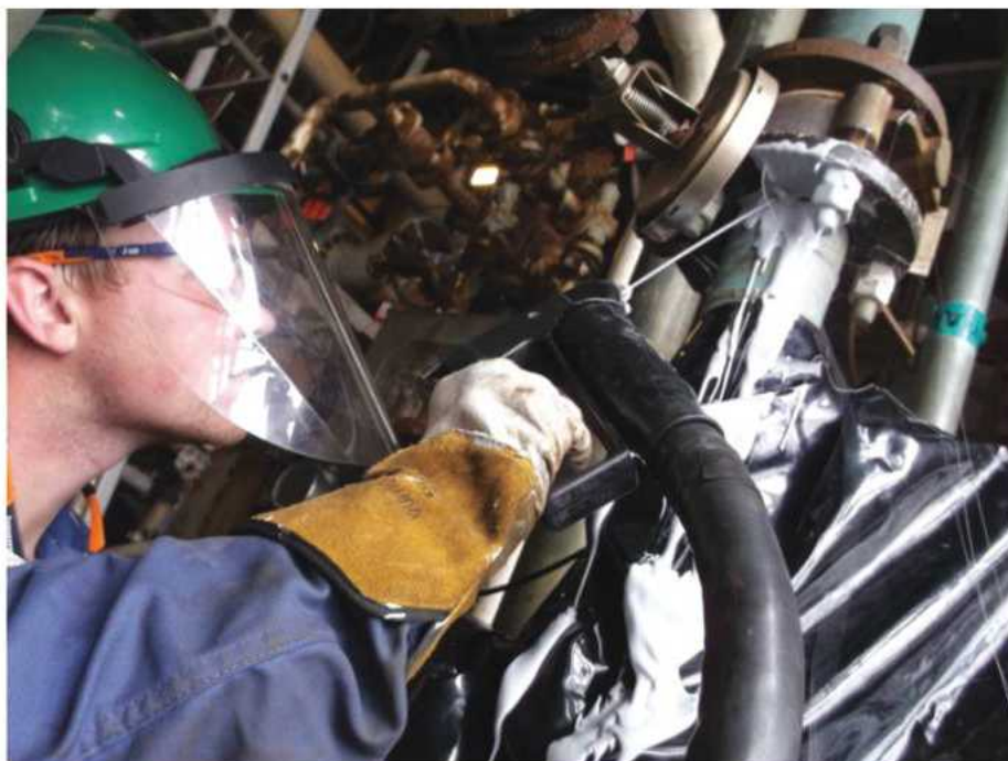
Keeping platforms going. Work on Piper Bravo by Oxifree. Photo from Oxifree.
