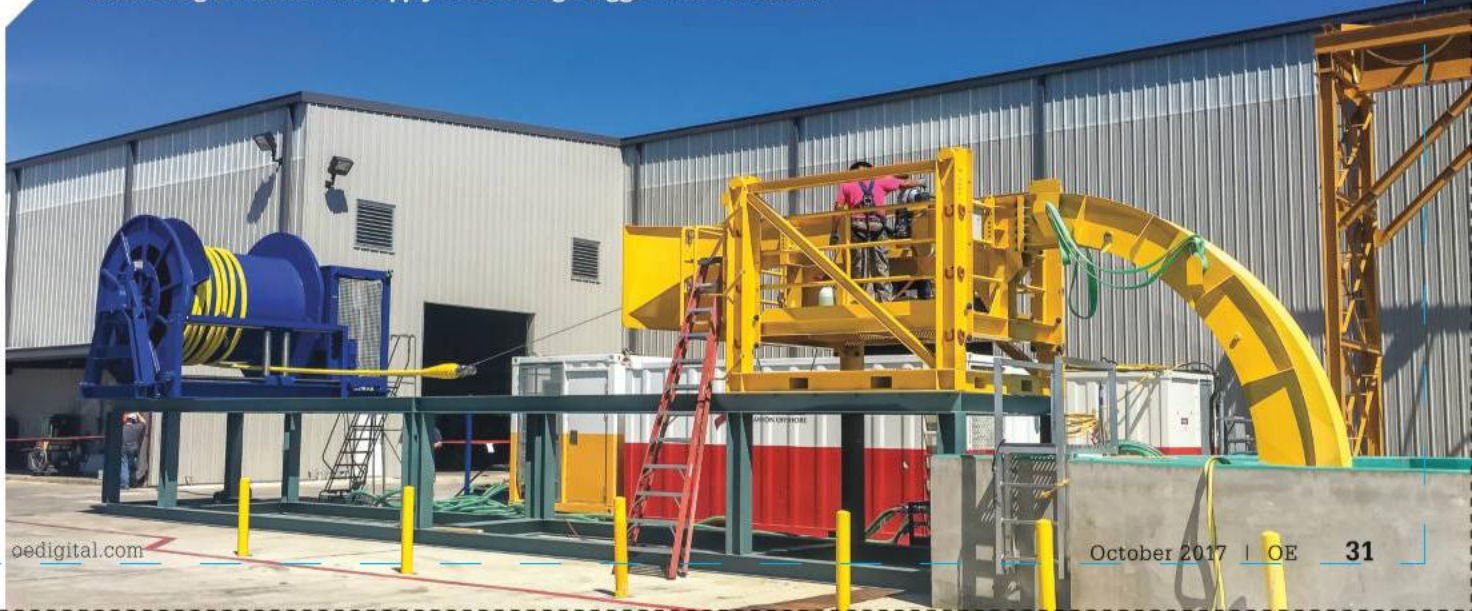
Interfacing between main supply hose through tugger winch on chute.
