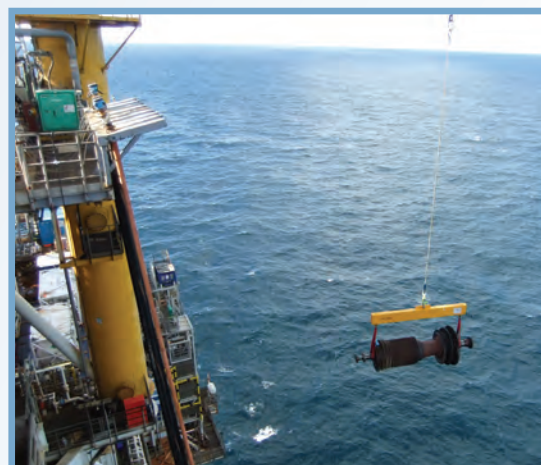
GE Frame 6 heavy industrial turbine rotor lift. Photos: Karl Grieve/Repsol Sinopec Resources UK.
