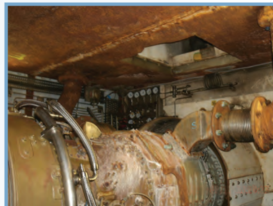
Rolls Royce Avon aero-derivative gas turbine.
